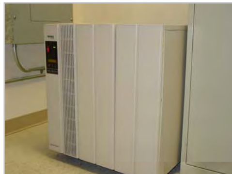
Our system is equipped with an Uninterruptible Power Supply (UPS) as a backup to protect all computers and electronic equipment including SenTrak.
