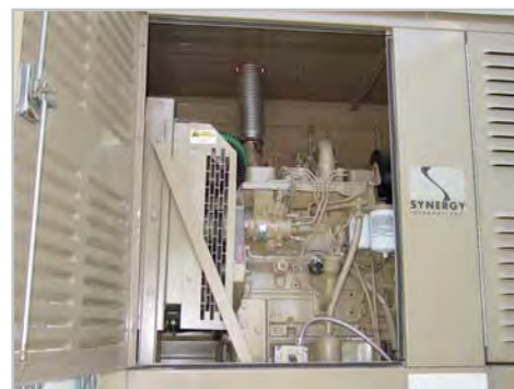
We have an on-site diesel generator to provide a minimum of ten (10) days of backup power without refueling.
