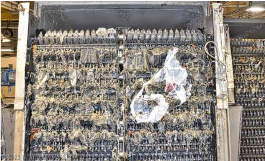
One of the skimmers at the water treatment plant. Not glamorous, but much needed upgrades to sewage and water treatment.
