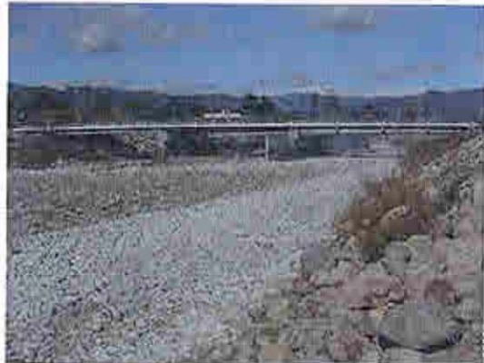
Figure 30. Ventura River looking northwest towards Santa Ana Blvd. Bridge 7.25 miles below Matilija Dam. 2-23-07
