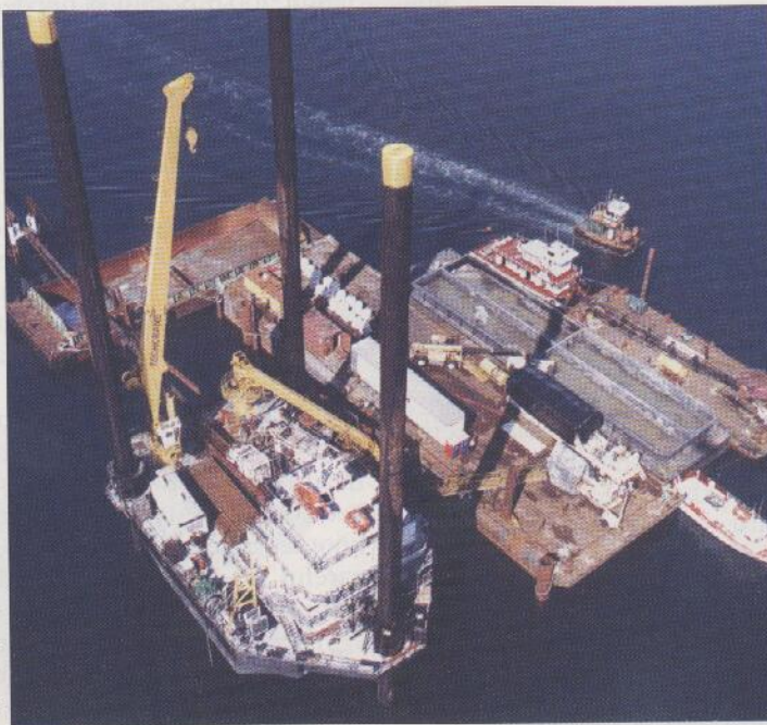
The Duke Energy Hubline project consisted of seven separate bores, showcasing the ability of HDD as an alternative to open-cut or dredging.
