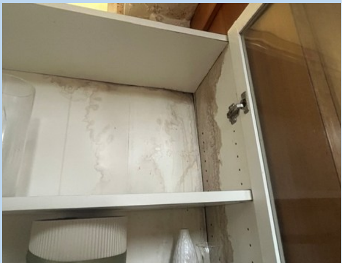
Significant leaks continue to cause damage to the children's room
