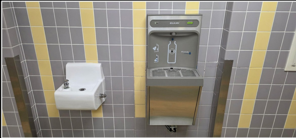
New water bottle filling station 1st Floor –East Wing
