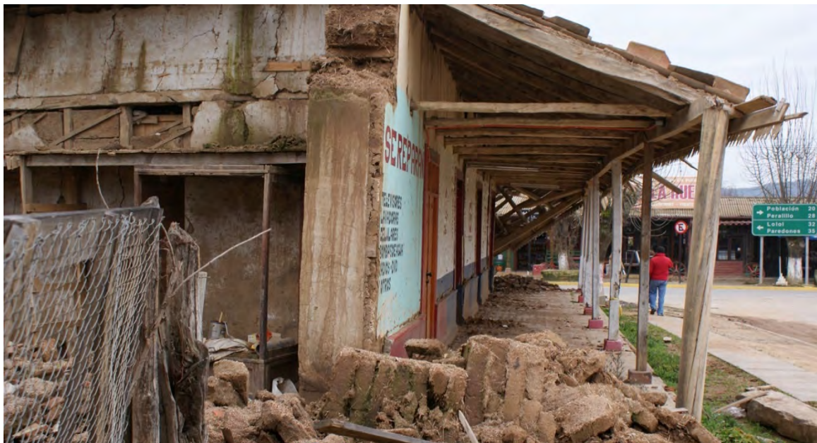
Figure 4: Dwelling severely affected by the 2010 Maule earthquake in Chile. Pumanque , Chile. April 2010 (Source: Author).
