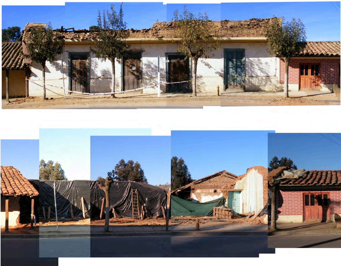
Figure 10: (above) Dwelling in Paredones after the 2010 earthquake. Above: before demolition. (Source: Muñoz, Alejandra).
