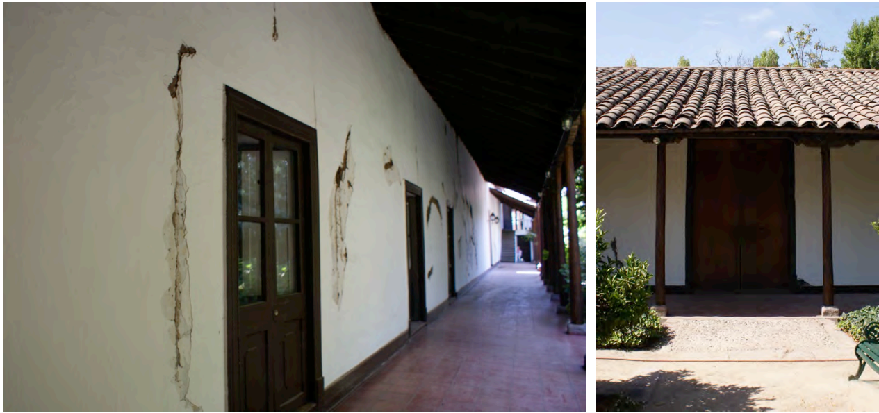
Figure 6 & 7: Casona Lo Contador , currently used as the School of Architecture of the Pontifical Catholic University of Chile. Photos taken one day after the 2010 earthquake, in which only superficial cracks can be seen. (Source: Author).
