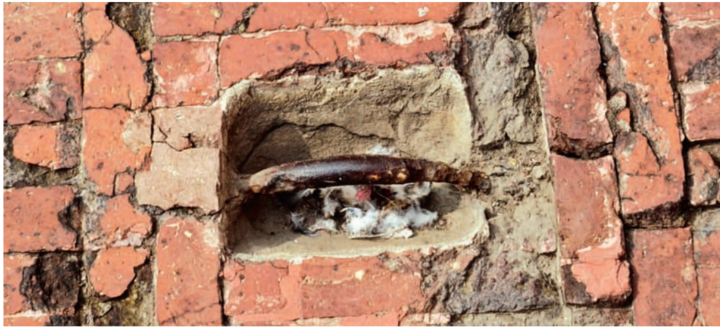
Puncturing of floor to accommodate fixtures such as metal hooks for tying shamiana ropes indicates the need for better and more appropriately located details.
