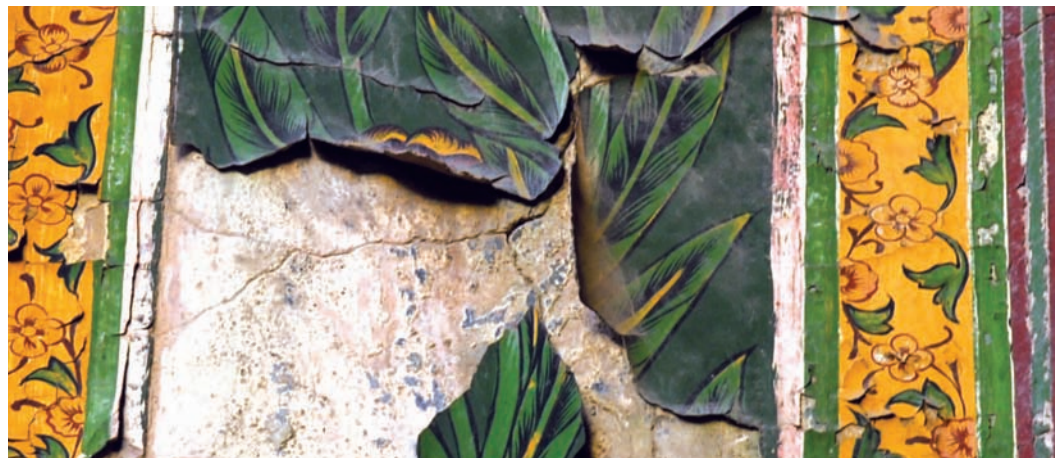
Peeling of upper coat of paint surface in the northern axial pavilion.
