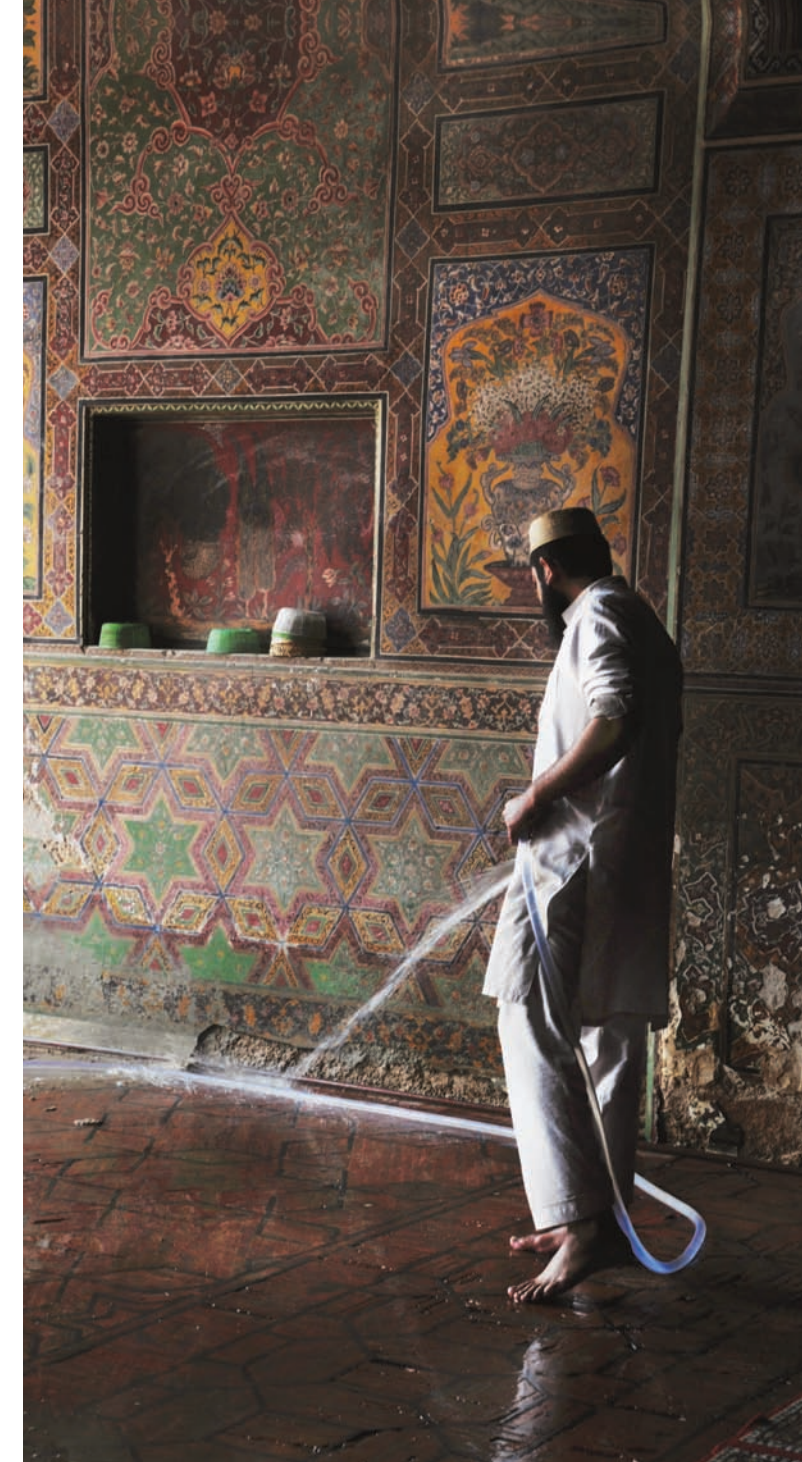
Above: Washing the floor with piped water under pressure, an activity unknown to the 17 th century builders of the monument. Note the damp rising up the wall and the plaster render with the precious wall painting breaking out under the force of the stream of water.
