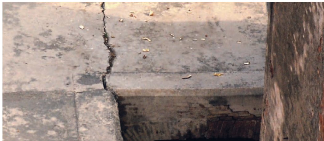
Major crack in the roof of the southern axial pavilion.
