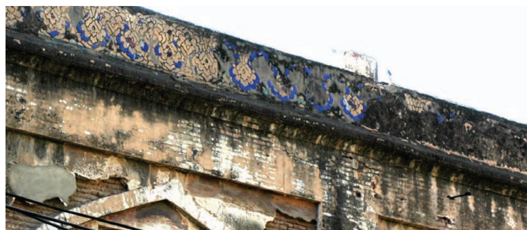
Advanced state of the deterioration of both mortar based external finishes such as faux brick and plain plaster render, as well as deterioration of crenellated tile work on the roof line of the north façade.
