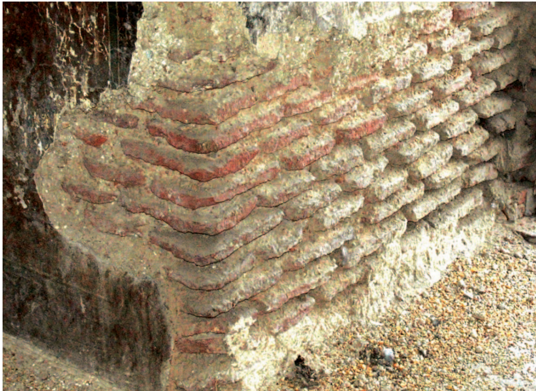
Erosion of mortar between the joints on the exposed surfaces of masonry.
