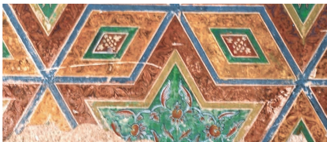
Peeling of the upper coat of surface render in the prayer chamber.
