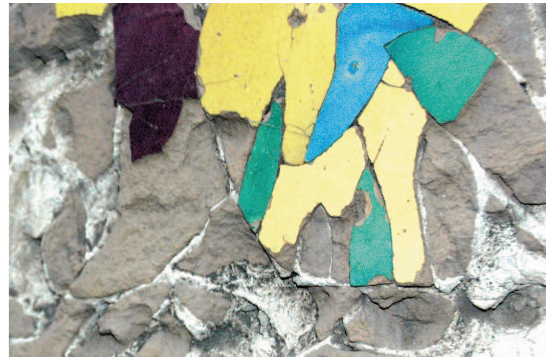
Advanced spalling of the core terracotta body of the tile.
