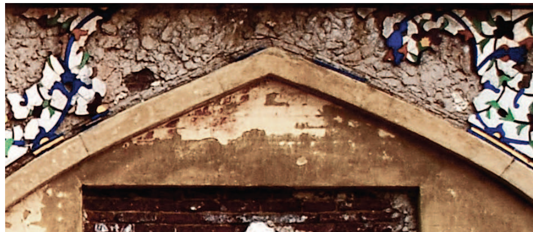
Partial loss of bond between tile and mortar.
