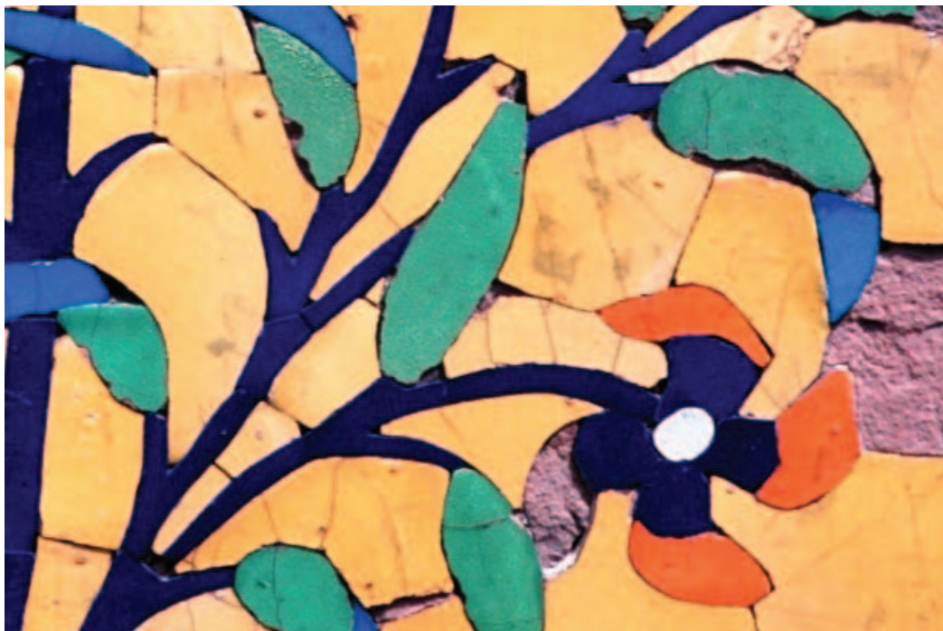
Pitting and spalling of thin layers of terracotta body of the tile. At this stage of deterioration, piece-meal replacement of sections of tile may be considered.
