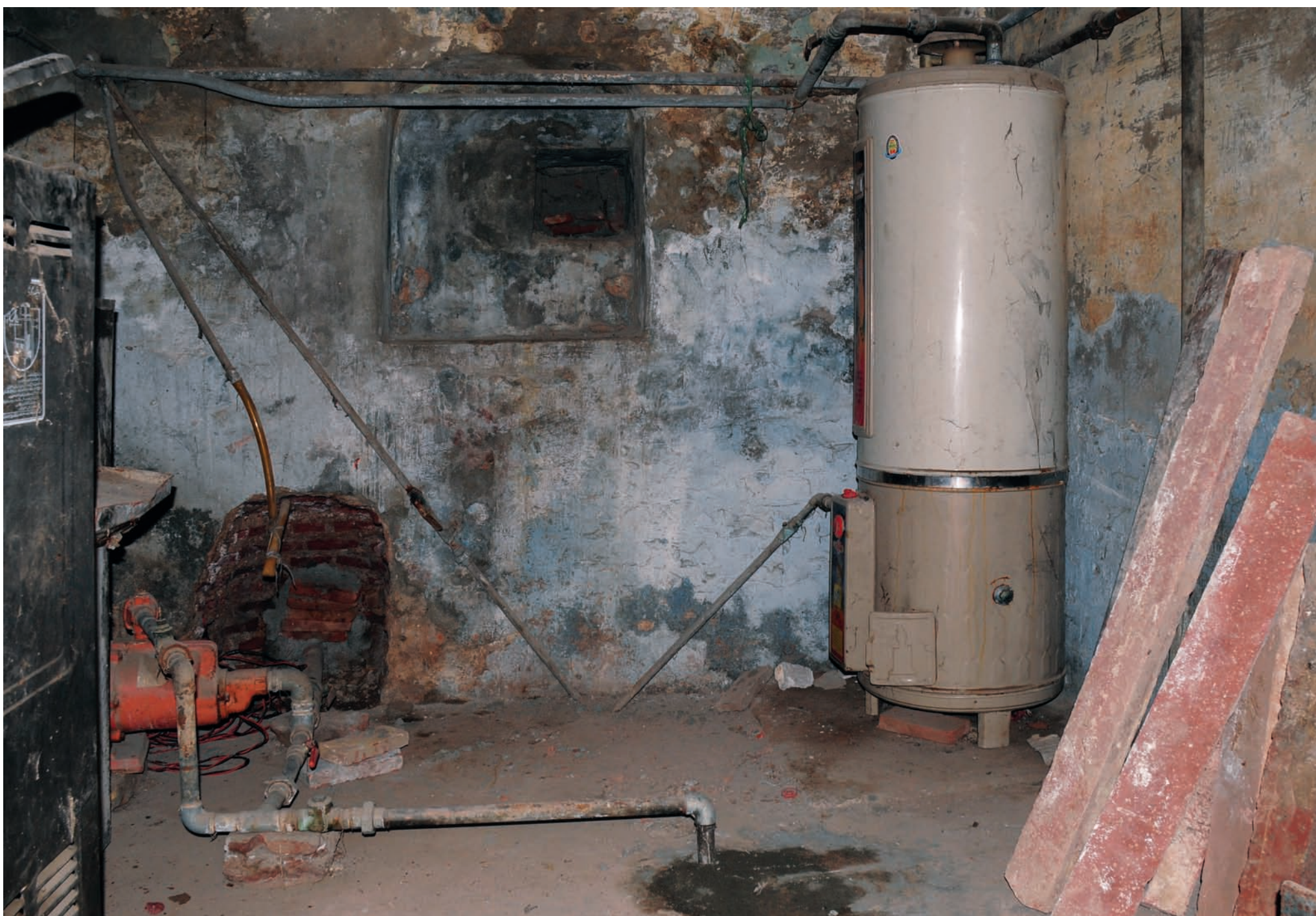
The hujra in the south-eastern corner of the mosque containing the water pump, water cooler and geyser.
