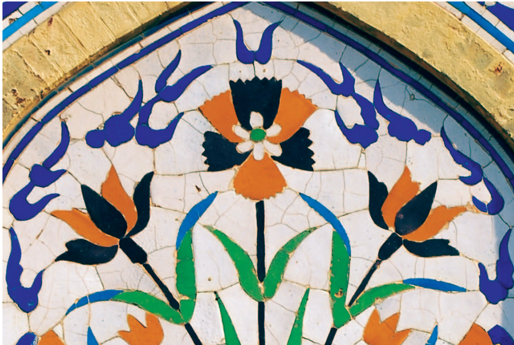
Hairline cracks on the glazed surface of tiles. These cracks are sometimes indistinguishable from the fine joints of the cut-to-shape tiles, but could be the beginning of more advanced weathering processes.
