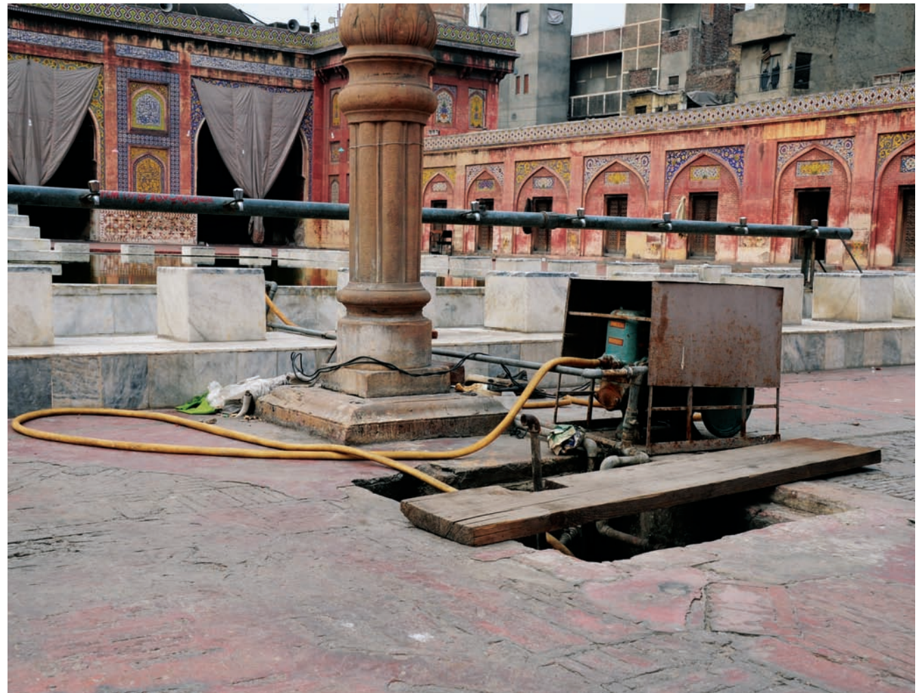
Above: Water supply pump positioned on the east side of the ablution pool - one of the first things visitors are confronted with on entering the courtyard from the entrance.
