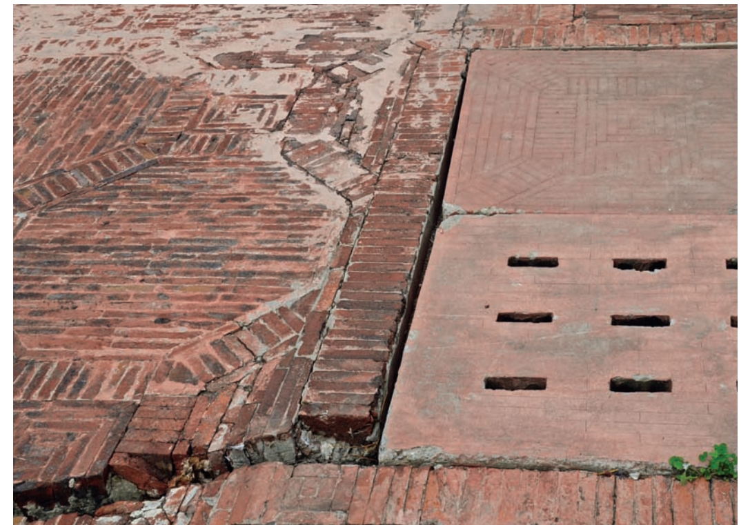
Puncturing of floors for installment of drains, drain outlets and gratings indicate the need for better and more sophisticated detailing.
