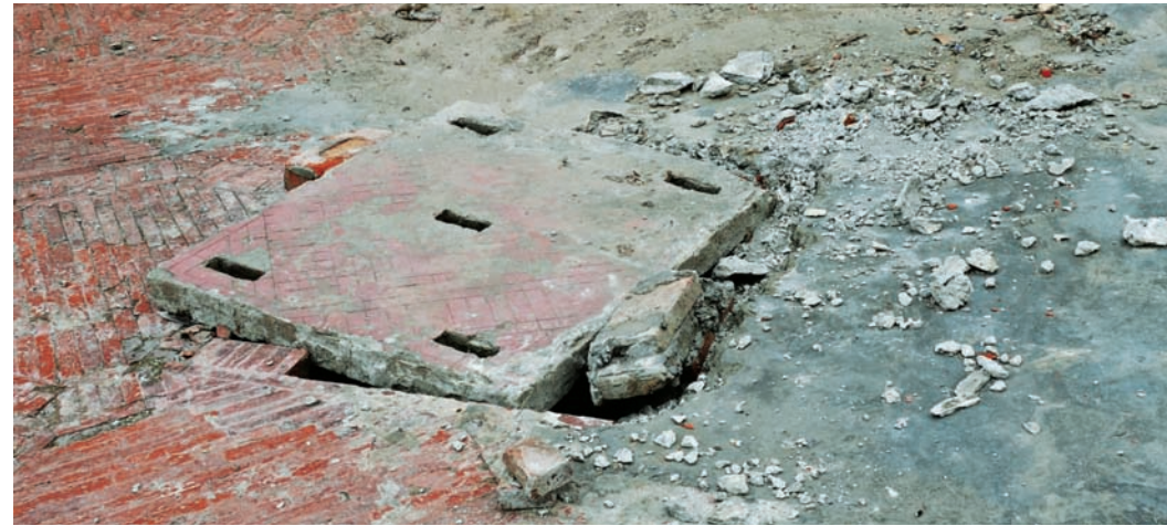
Poor detailing of waste and storm water disposal grating.
