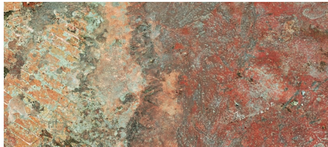
Inappropriate use of materials to repair floor - in this case coloured cement / sand or coloured lime render.
