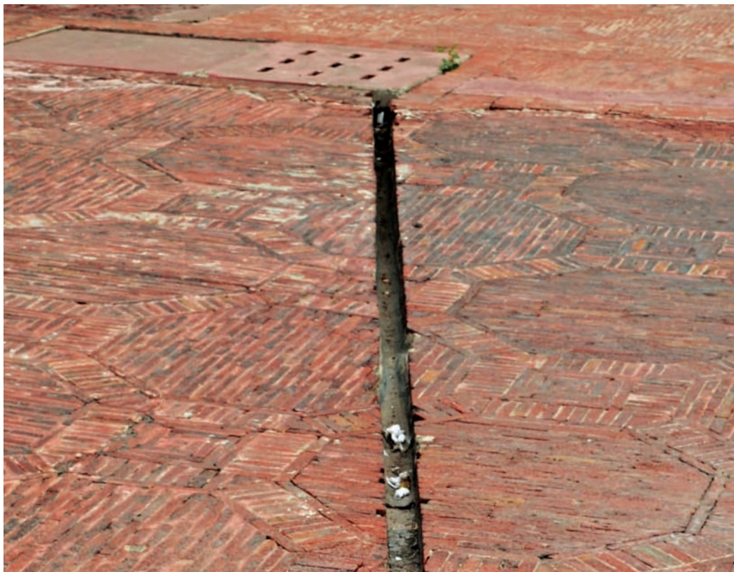
Cutting up the patterned floor to accommodate a collector drain. A better and well distributed system of under floor drains is required.
