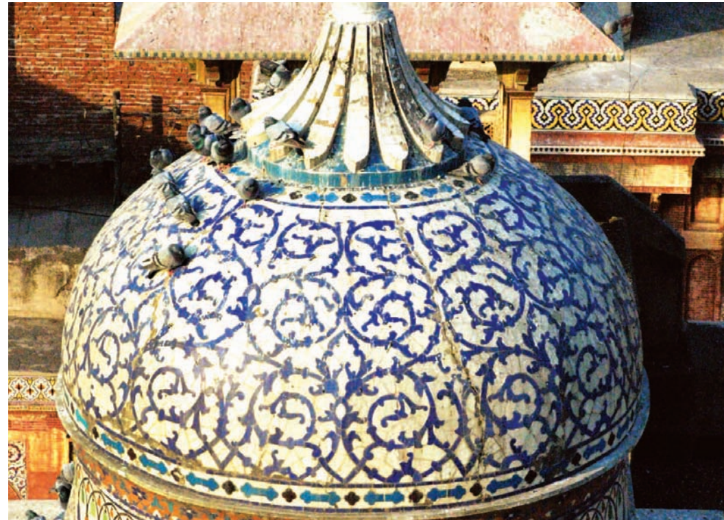
Major crack in one of the domes of the chhatri above the entrance iwan.
