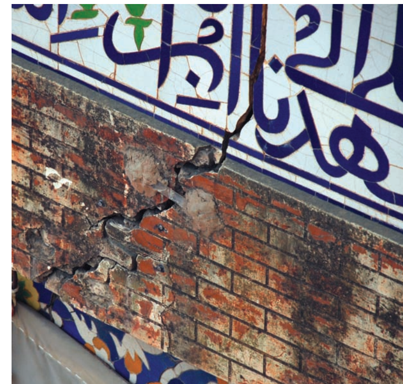
Top: The crack in the apex of the arch forming the southern most entrance into the prayer chamber.
