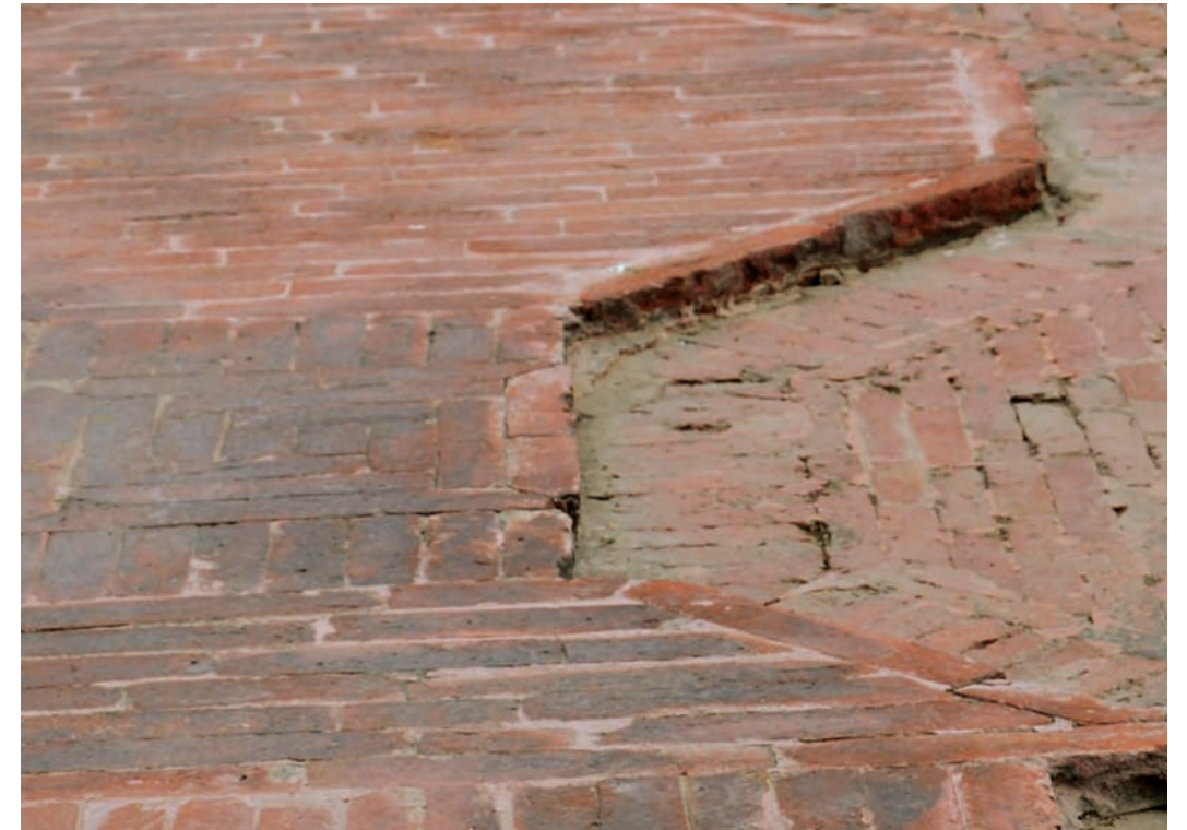
Subsidence and inadequate repair at different levels.
