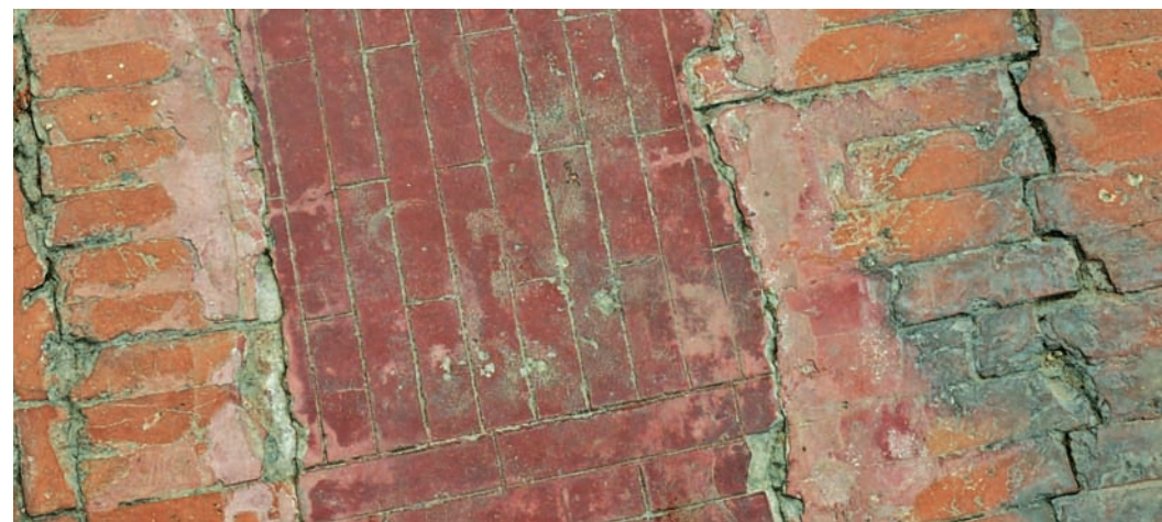
Brick and fake brick markings on cement / sand or lime / sand renders create an unsatisfactory appearance. Note the subsidence crack on the right of the photograph.
