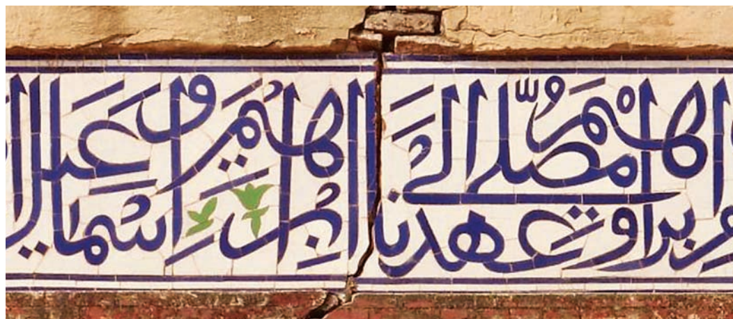
Major crack in the wall above the northern most archway of the prayer chamber.
