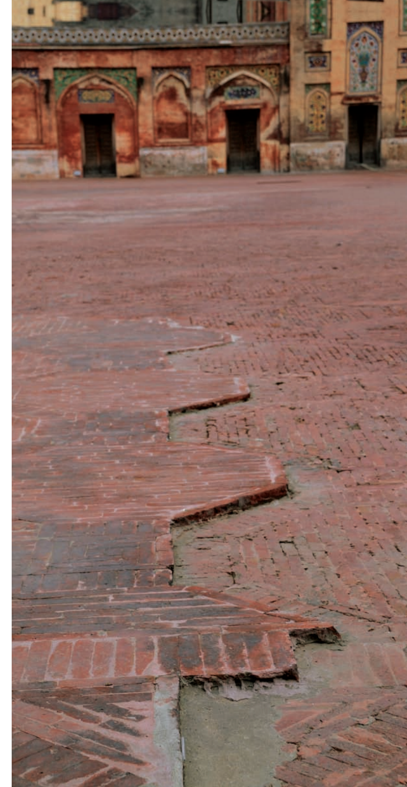
Above: Subsidence and floor repair in the north-west corner of the courtyard has created different levels with badly finished edges.
