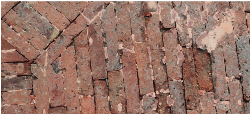
Erosion and disintegration of brick with surface wear.
