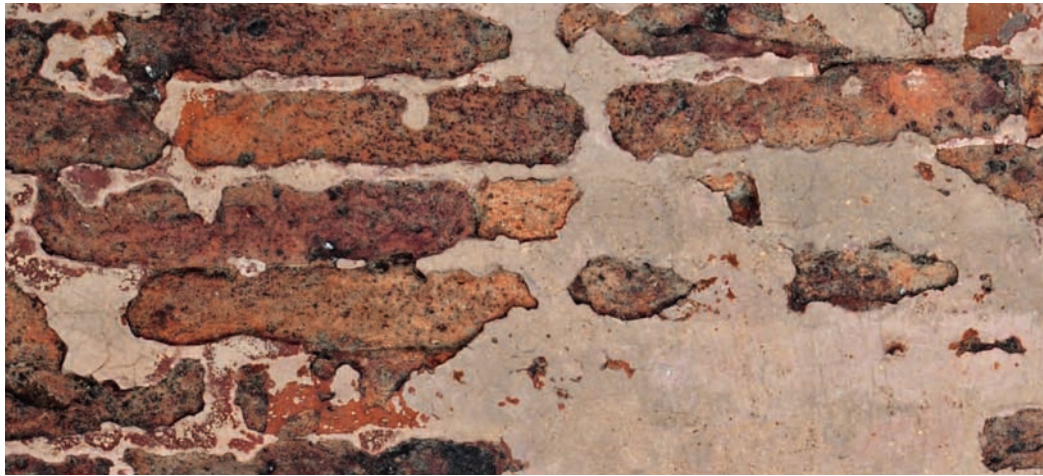
Inappropriate use of cement/sand renders and over-grouting between bricks.
