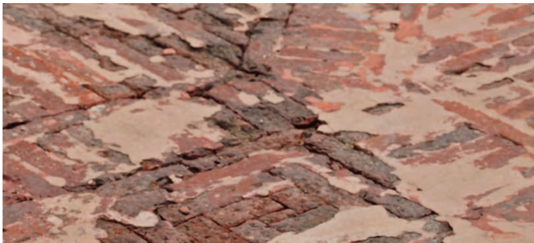
Faster rate of erosion of bricks with the inappropriate use of cement/sand renders used to achieve a water repellent surface.
