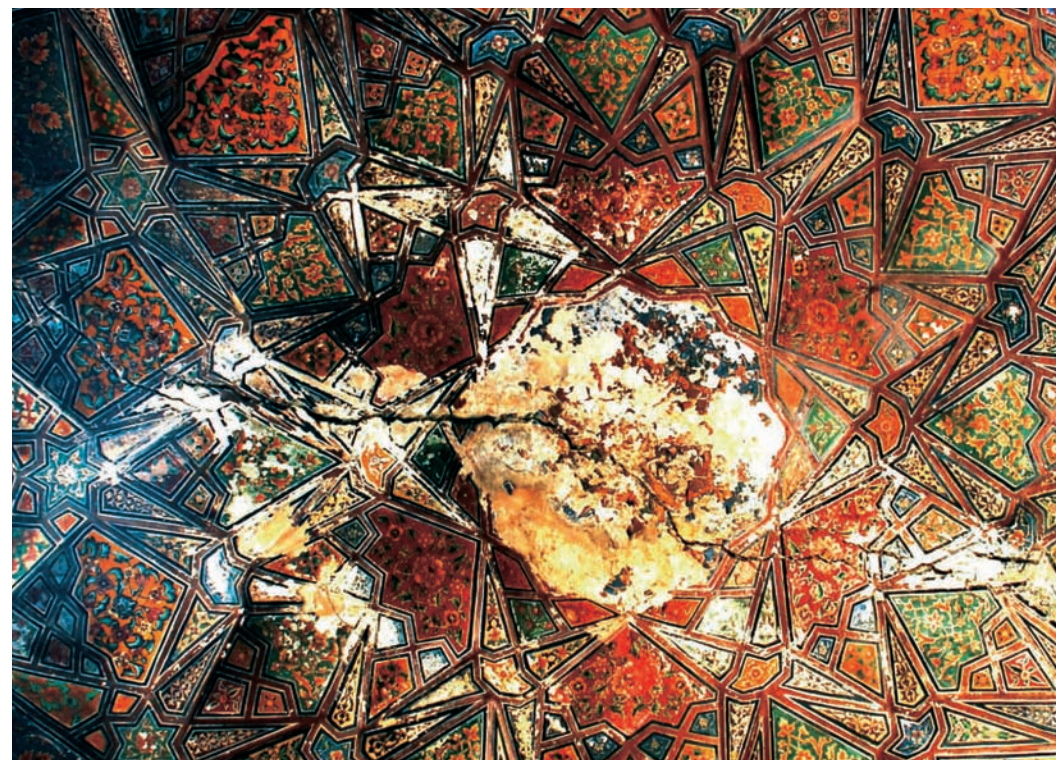
Major crack in the vault of the northern most archway of the prayer chamber.
