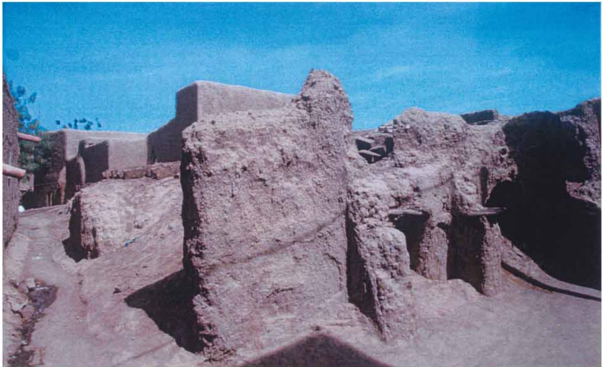
Above: A badly deteriorating house in need of reconstruction.
