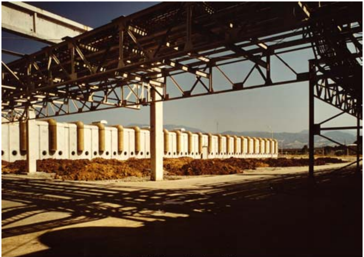
Plant building with pipe bridge
