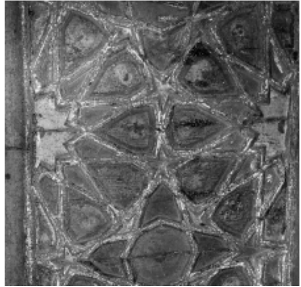
Sabil Kuttab: decorated lower ceiling before cleaning
