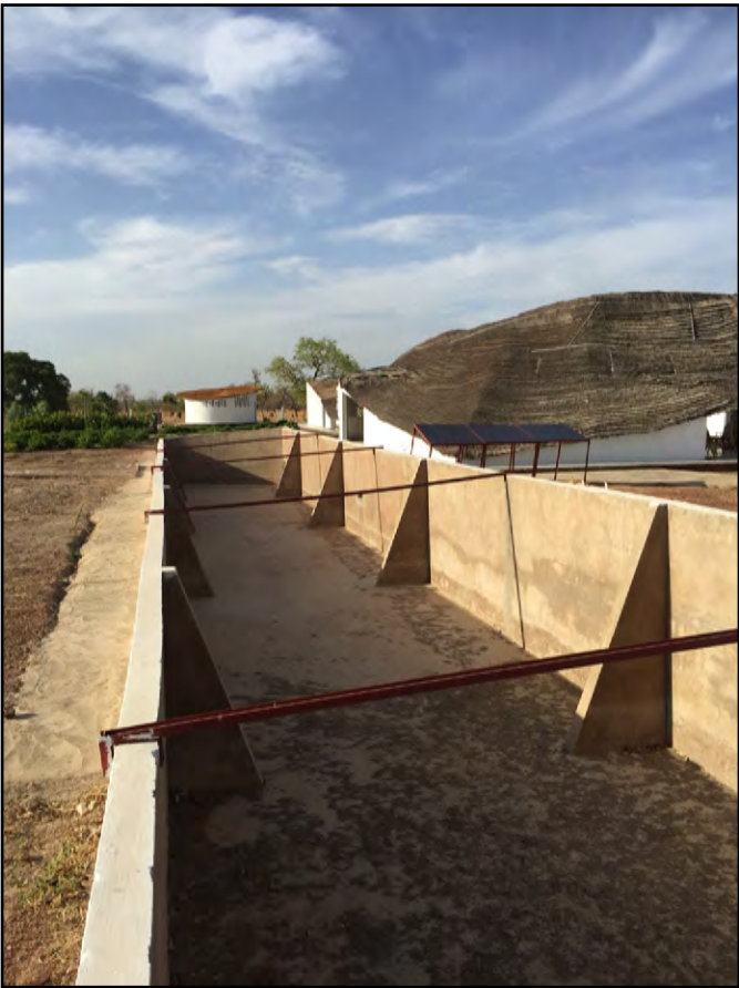
One of the main features of the design is the rain water harvesting roof, which fills two underground tanks water reservoirs and provide irrigation water for 7 months/year. One of them suffered from poor reinforcement in the concrete walls but is now been tendered to with a complete overhaul of the reinforcement.
