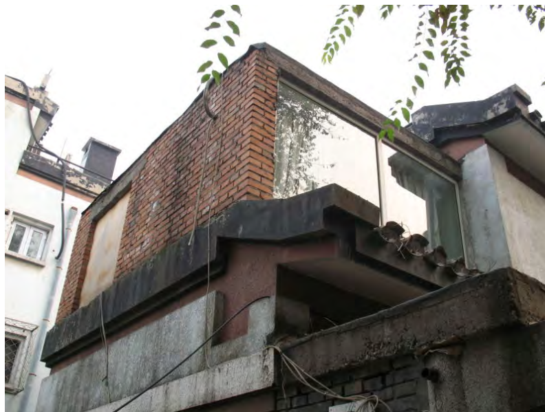
Figure 11. Although the roof-level enclosure adds interior space, it creates visual disorder, Juer Hutong new courtyard housing (Source: Author).
