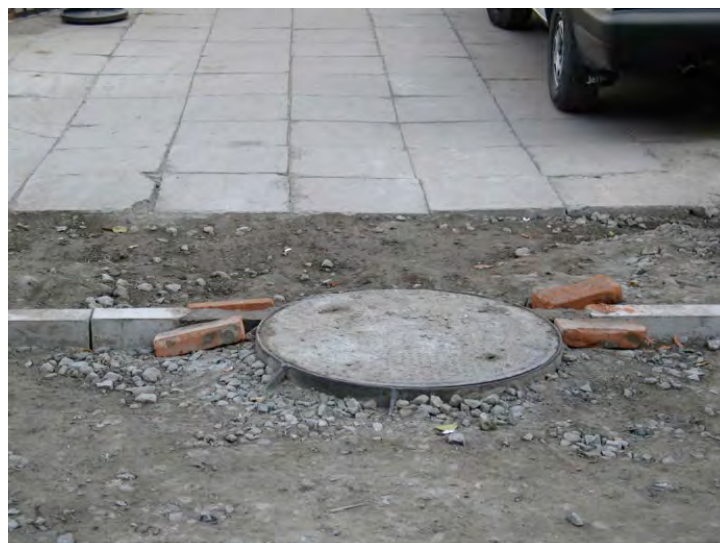
Figure 15. The road of Juer Hutong after reconstruction is higher than the courtyard level, forcing rainwater to flow back into the yards (Source: Author).
