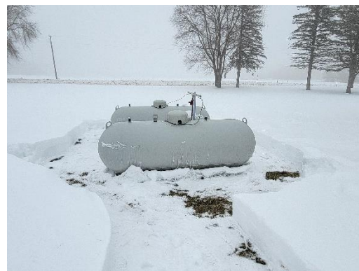
#1 Properly cleared access to tanks
