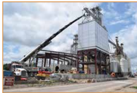
A 285-ton crane was brought in to set up new pellet mills and conditioners as part of the feed mill expansion.
