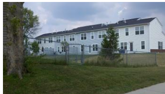
Needs weeded at fence line
