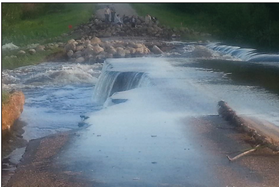
The Highway to Atwater was one of the many roadways destroyed by rising waters after a torrential rainstorm hit the south-east area of Saskatchewan on June 28-29. Photo by Crystal Johnson
