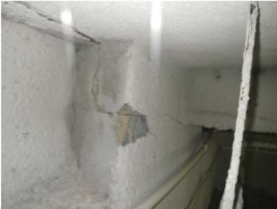
Photo 09 - shotcrete and cracks
