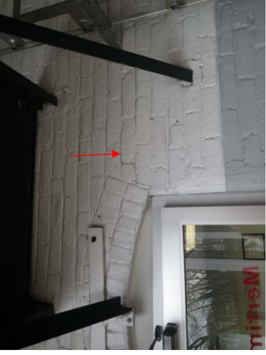
Stepped crack at interior brick wall
