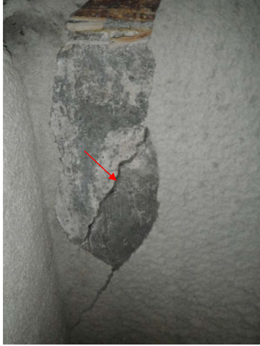
Diagonal crack in foundation wall
