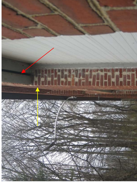
Slight rotation at top of jamb + lintel separation
