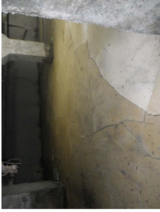
Concrete infill with surface cracking
