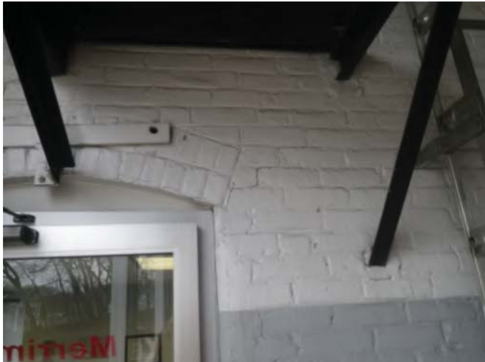
Photo 04 - Int stepped crack
