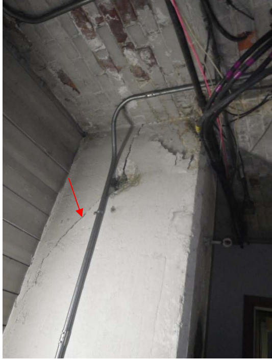
Typical crack in steel beam encasement
