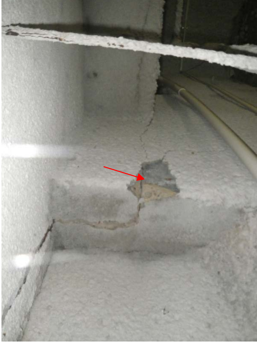
Concrete layering at wall + beam – note cracking
