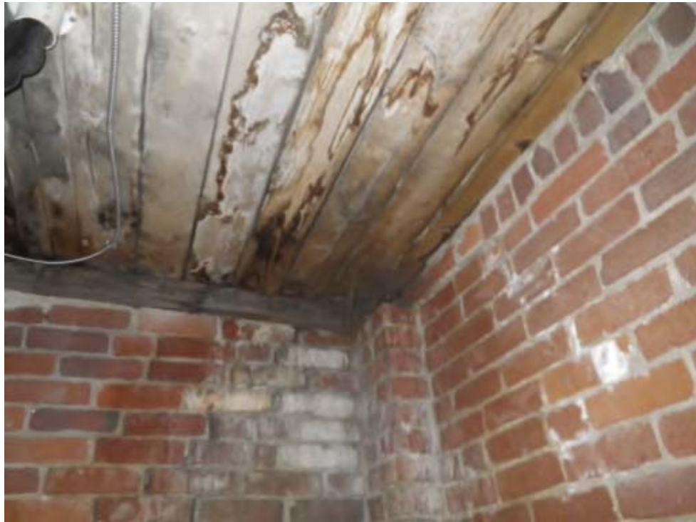
Photo 15 - rot and crack
