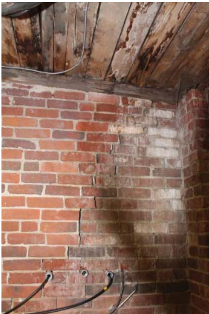
CONDITION AT INTERIOR WALL (POLICE DEPARTMENT)
