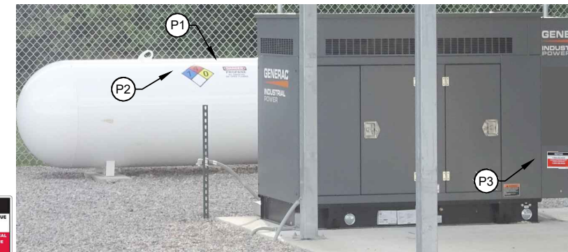
FIGURE 7 - PROPANE TANK & GENERATOR SIGNAGE
