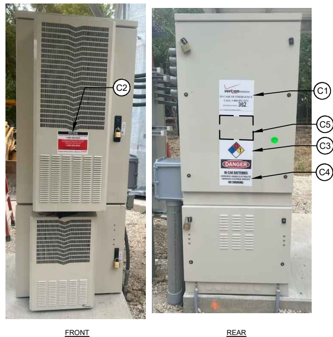
FIGURE 1 - EQUIPMENT CABINET SIGNAGE
