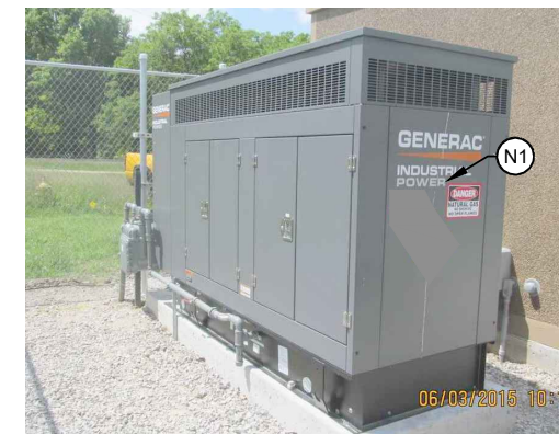
FIGURE 8 - NATURAL GAS GENERATOR SIGNAGE
