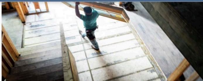
A contractor carries a new window inside a West University house Houston Chronicle Staff
