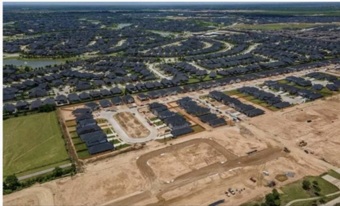
The beginning stages of construction in a new development in Conroe. Mark Mulligan/Houston Chronicle
