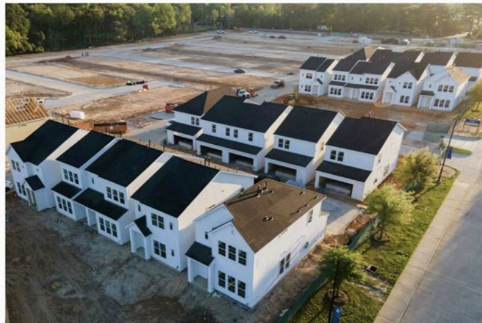
Construction continues in a new community of multi-family homes in The Woodlands. Houston Chronicle Staff
