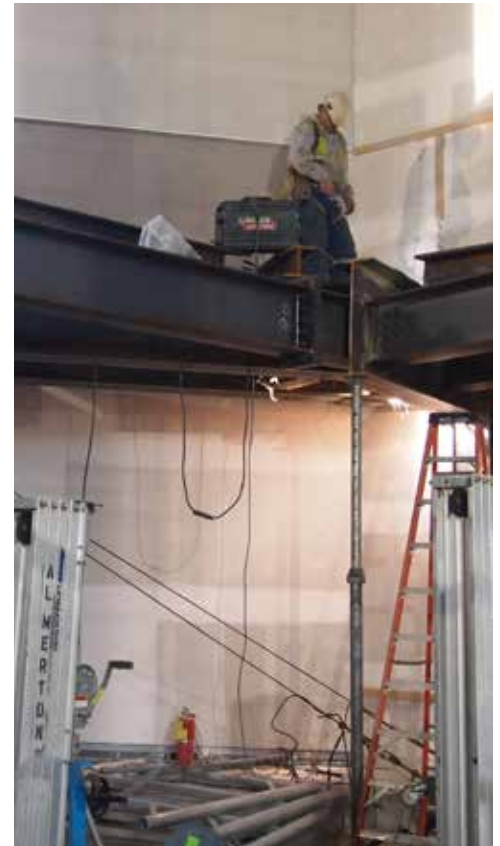
A Forrester Construction worker evaluates his progress on expanding the balcony level all the way to the front of the Charles E. Smith Sanctuary.
