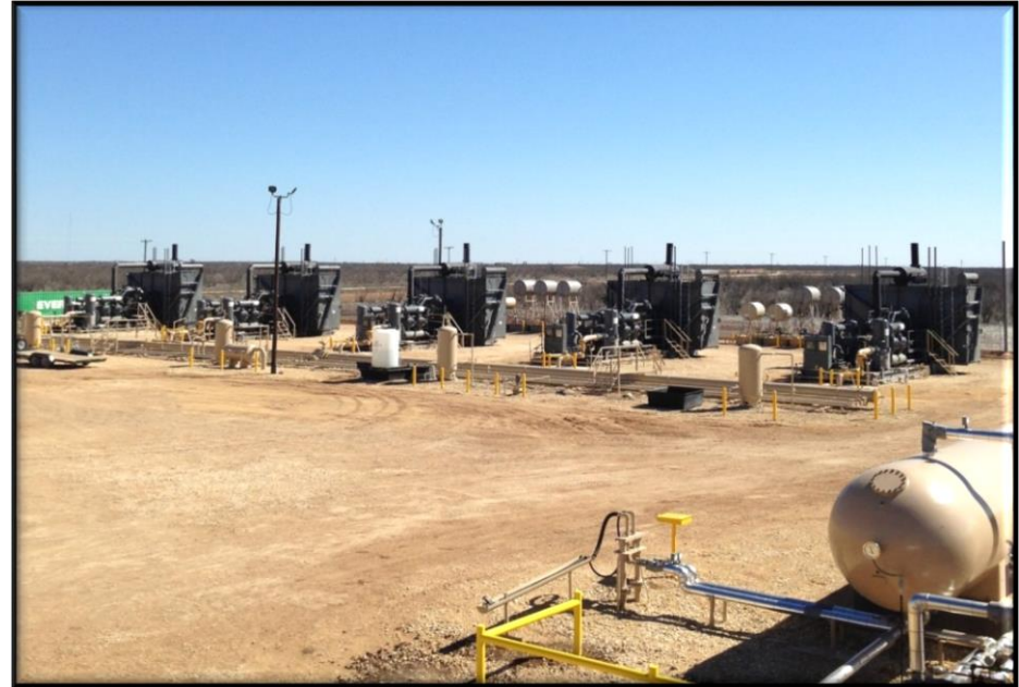
Reagan North Centralized Compressor Facility
