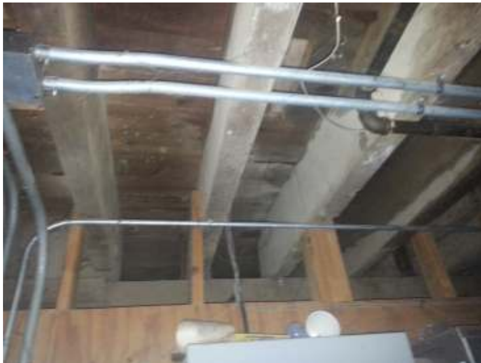
PICTURE 6: THE FLOOR JOISTS AND SUBFLOOR AND OTHER SURFACES THROUGHOUT BASEMENT ARE COATED WITH FUNGAL GROWTH.
