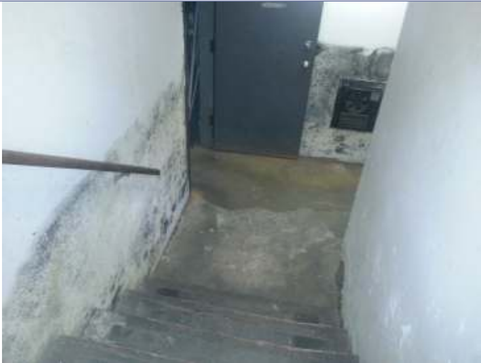
PICTURE 3: FUNGAL GROWTH FROM WATER SOAKING UP THE LOWER SHEET OF WALL FINISH.
