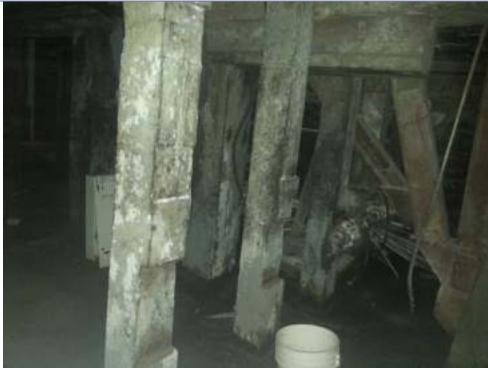
PICTURE 5: THE PILLARS AND OTHER SURFACES IN THE BASEMENT ARE COATED WITH FUNGAL GROWTH.
