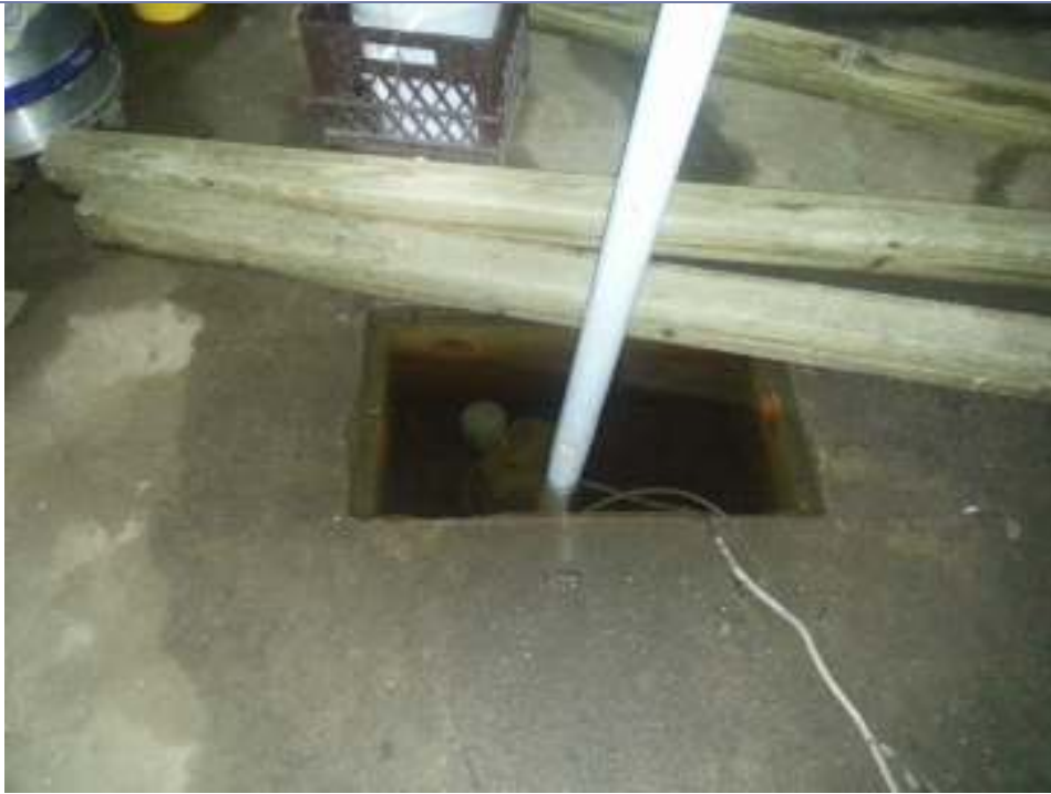
PICTURE 7: SUMP CROCK FILLED WITH WATER.
