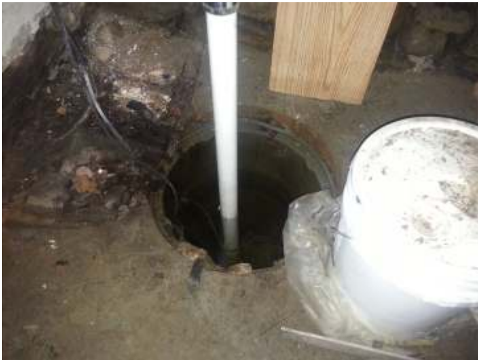
PICTURE 8: SUMP CROCK FILLED WITH WATER.
