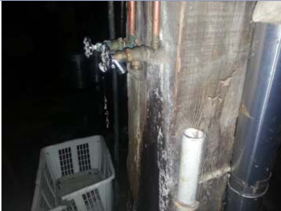
PICTURE 9: WATER DRIPPING FROM A SPGOT IN THE BASEMENT.
