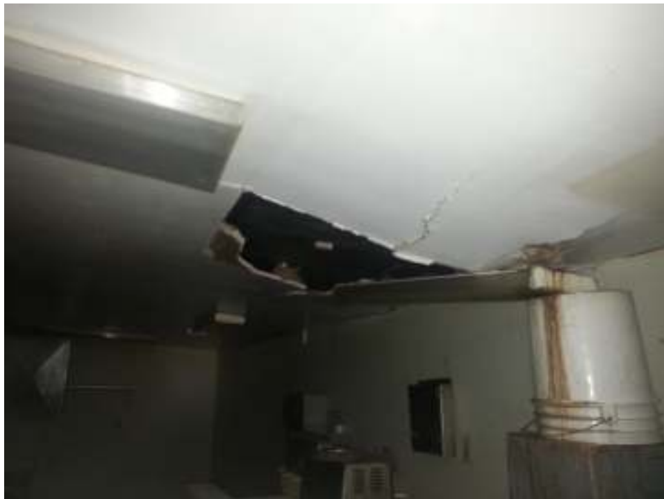
PICTURE 14: DAMAGE TO KITCHEN CEILING.
