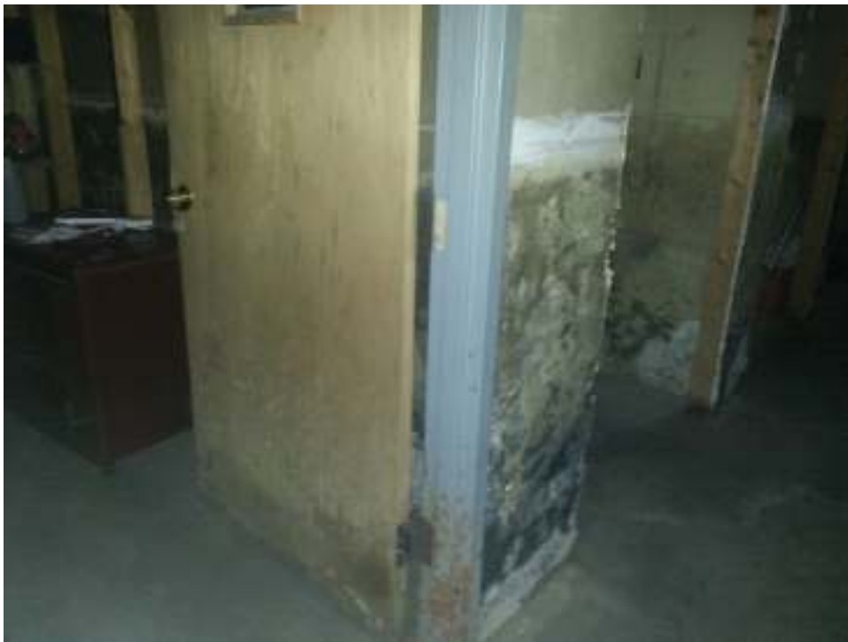
PICTURE 4: FUNGAL GROWTH FROM WATER SOAKING UP THE LOWER SHEET OF WALL FINISH.
