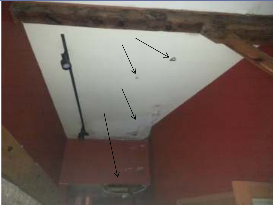
PICTURE 15: DAMAGES TO CEILING OF HALLWAY.
