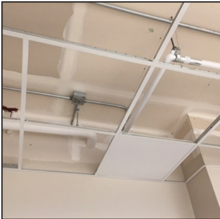
Ceiling: Grid work has been completed and ceiling tiles are being installed.
