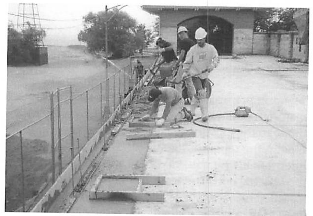
Figure 7. Placement of architectural concrete along the projecting edge of the upper terrace. The concrete was placed against formwork with a concrete retarder and then hand finished to match original concrete. (WJE)
