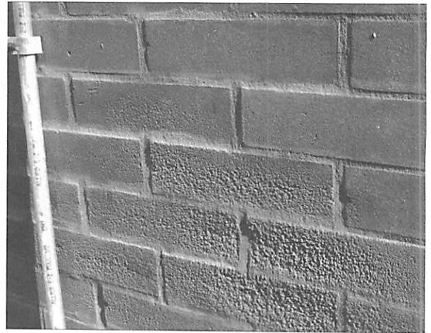
Figure 2. Inappropriate cleaning can irreparably damage building materials, such as the etching of this brick facade. (WJE)
