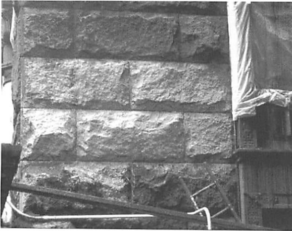
Figure 1. Successful cleaning can remove harmful deposits and enhance the appearance of historic buildings. (Wiss, Janney, Elstner Associates, Inc.)
