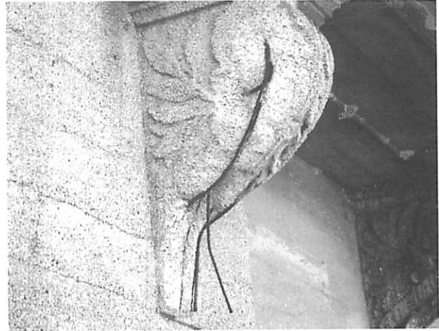
Figure 4. Severe deterioration of a concrete ornamental bracket below a balcony. The deterioration was due to corrosion of embedded reinforcing steel. (WJE)
