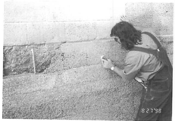
Figure 6. Craftsman placing and finishing repair concrete in a mock-up area. The craftsman developed techniques to maintain an inconsistent aggregate exposure to match the variability in the original adjacent concrete. (WJE)
