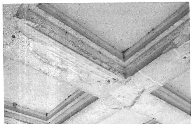
Figure 5. Typical concrete spall in coffered-ceiling beam in the colonnade. The corroded reinforcing steel was coated with epoxy paint for short-term protection. (WJE)
