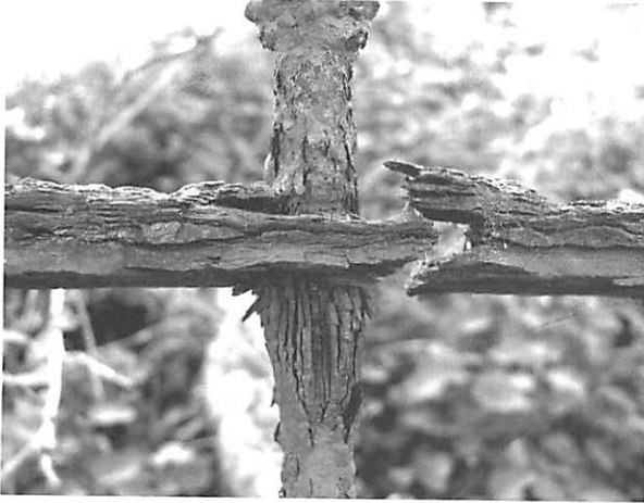
Figure 4. Conservation challenges indeed—wrought iron delamination in a marine environment, Stornoway, Western Isles (Copyright, D.S. Mitchell)
