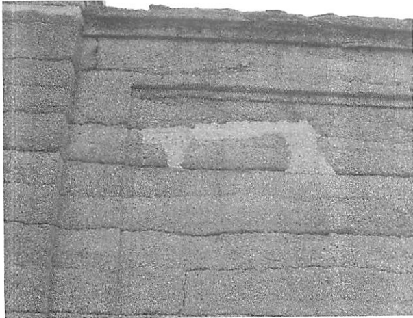
Figure 3. Wall construction of the Beach House with lift lines between concrete placements. Note the intentional inconsistency of the placement and variable aggregate exposure. (Wiss, Janney, Elstner Associates, Inc.)
