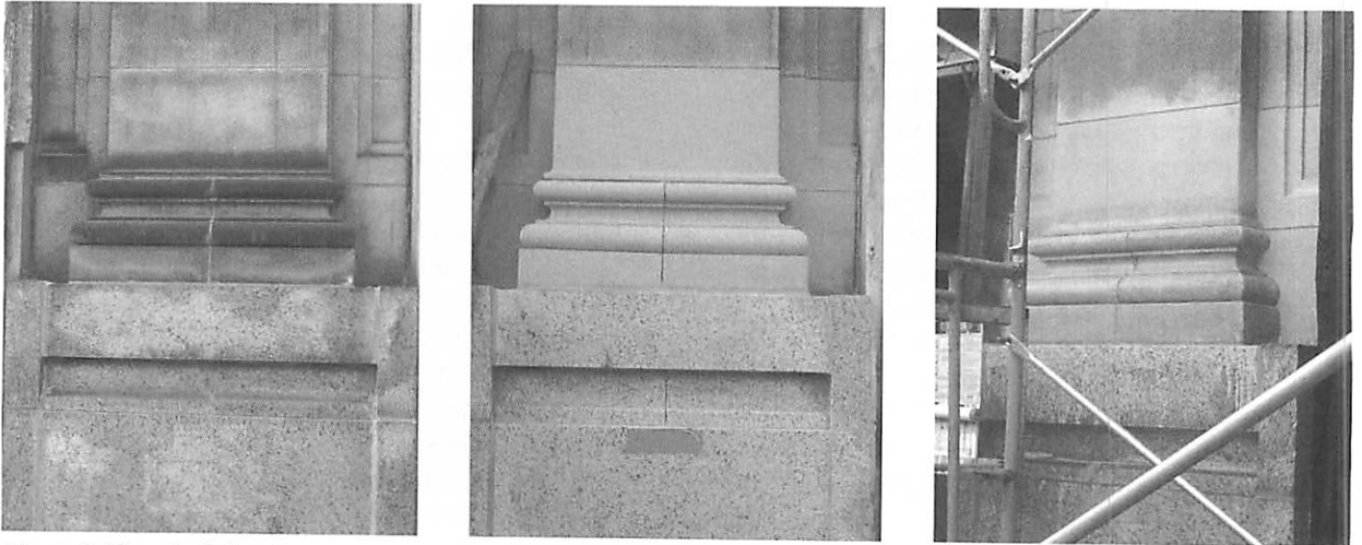
Figure 6. Chemical cleaning was used on this terra cotta and granite facade in Chicago to remove general surface dirt from water runoff and air pollution. At left, the original appearance of the facade. At center and right, field samples of two different chemical cleaning products. An examination of the sample at center with a field microscope suggested that damage to the terra cotta substrate could occur; therefore, the product used for the sample at right was selected to clean the building. (WJE)
