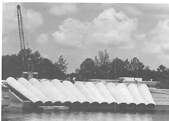
Figure 2. The Mermaid Theater under construction in 1958 (Weeki Wachee Springs, LLC, Archive Collection)
