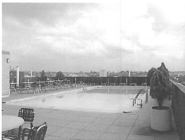
Figure 6. The rooftop pool of the Seville is still used today. The pool’s original tile remains, as does the surrounding wood fencing. The roof was replaced in the late 1990s, during which the pool deck was repaved. (L. Van Damme)
