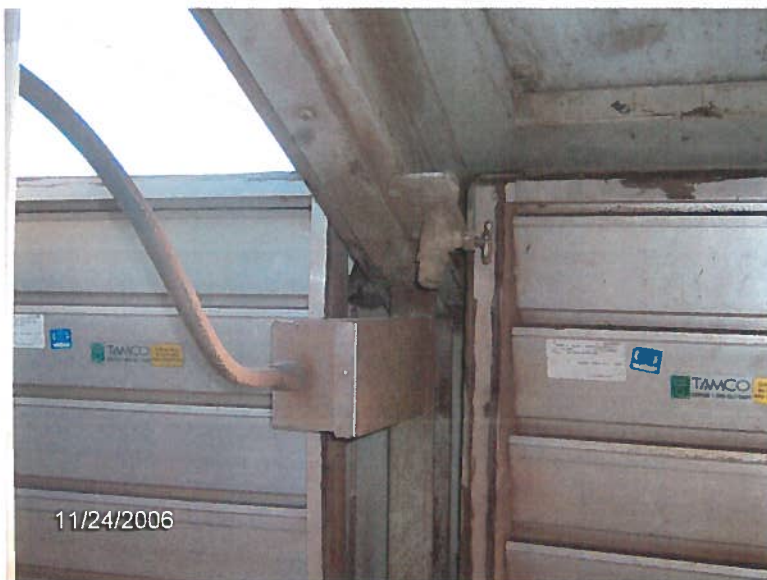
Figure 10: Drainage System Flushing Valve at Apex Louvers
