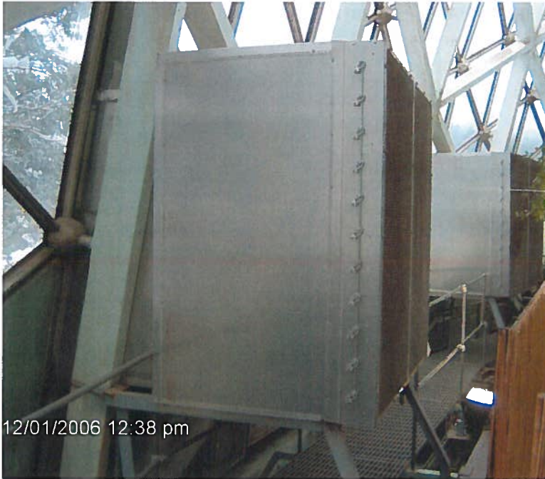
Figure 12: Wall Exhaust Fans for Summer Ventilation
