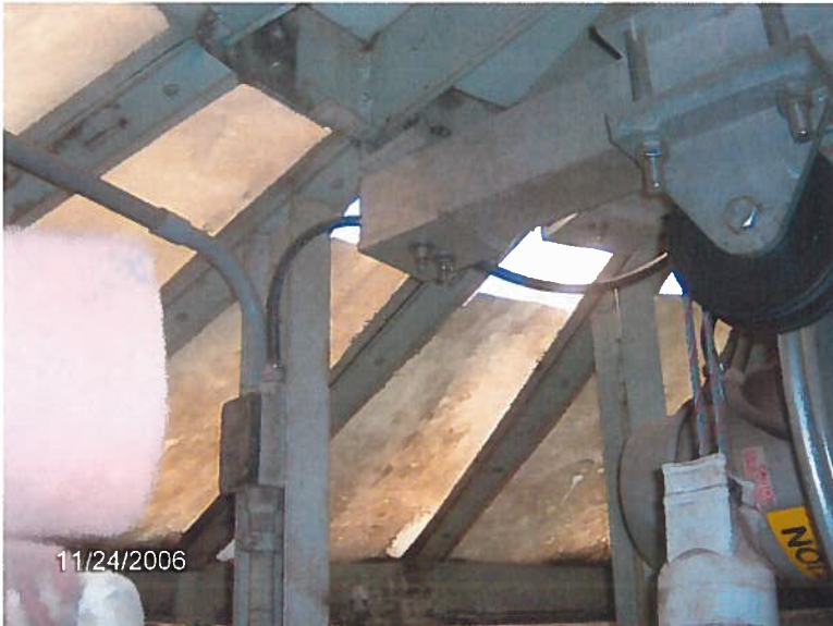
Figure 9: Stained Translucent Panels above Mechanical Equipment
