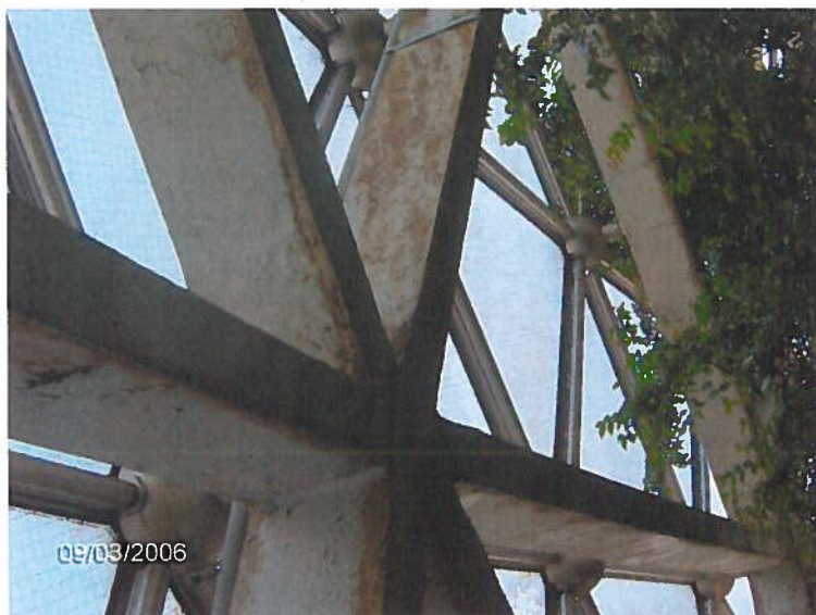
Figure 5: Typical Paint Peeling and Staining on Concrete Frame
