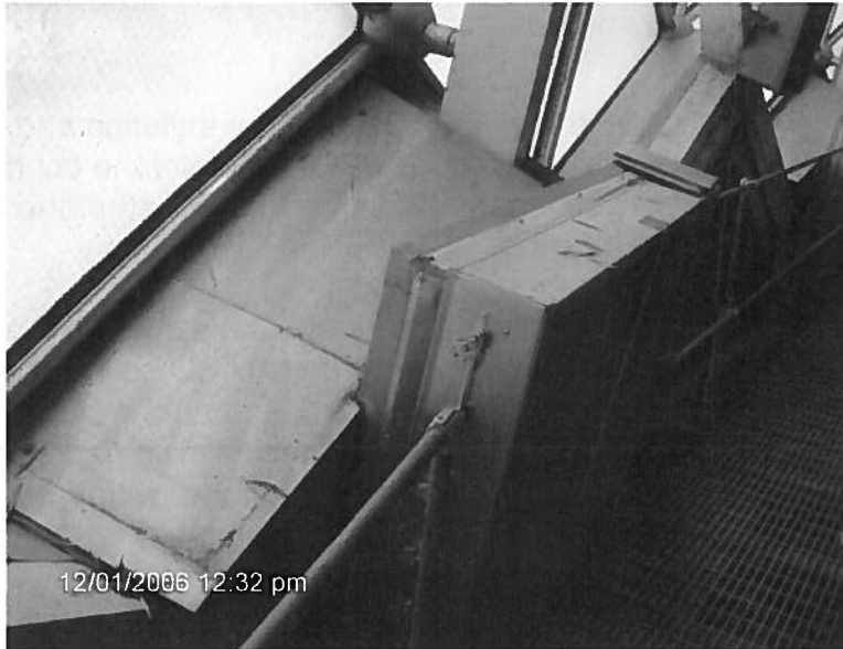
Figure 11: Typical Summer Air Intake (SAI)
