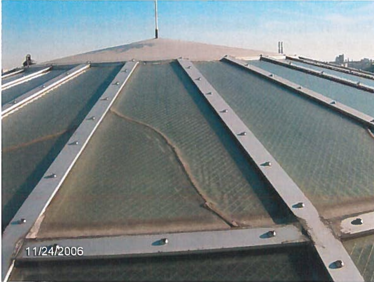
Figure 8: Damaged Glass Panels at Show Dome Apex
