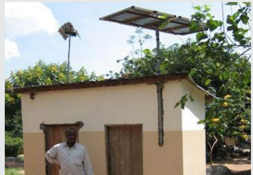
A solar panel installed on a villager's home in Africa Source: http://www.ashdenawards.org/winners/zara
