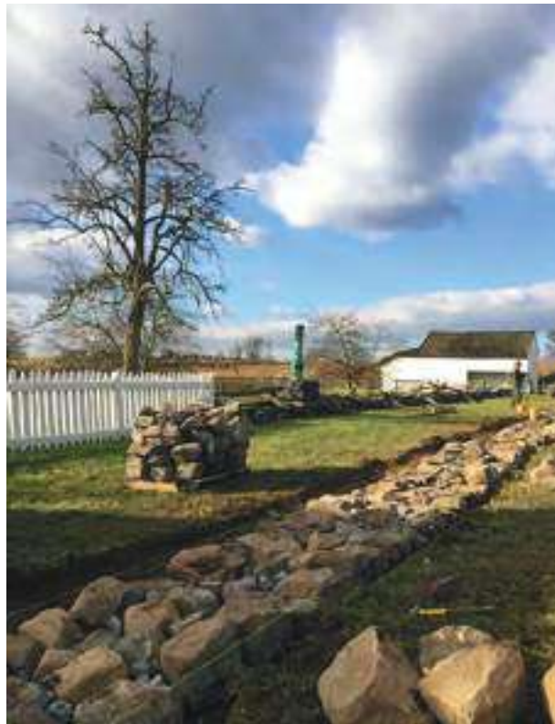
The stone wall along the Leister Farm Lane was constructed in December 2016. PHOTO AND CAPTION COURTESY GETT.
