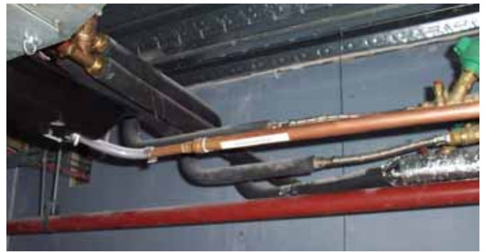
Figure 5.2 Condensate disposal pipework from drain tray
