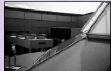
Condensors installed to serve the computer room chillers are located very close to the inlets serving the office chiller.
