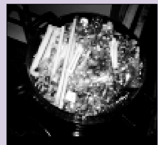
Evidence of the high rate (in reality up to 40 every month) at which the metal halide lamps need to be replaced. Each lamp costs £25.
