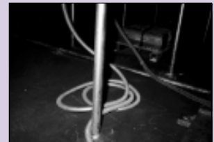
Lighting ballasts in the floor plenum are believed to be responsible for a 1°C hike in supply air temperature.
