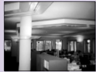
The general office area. Some perimeter chilled beams are located in the atrium extract path.
