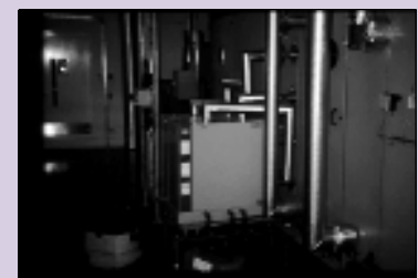
One of the rogue humidifiers which often runs in summer to replenish the moisture that is removed at the cooling coil.
