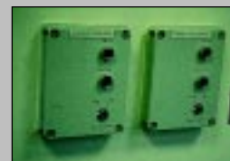
Top marks for the good window controls...
