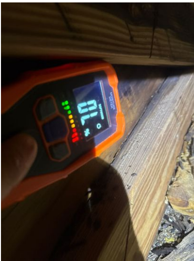
Unsatisfactory (attic water stain tested WET)
