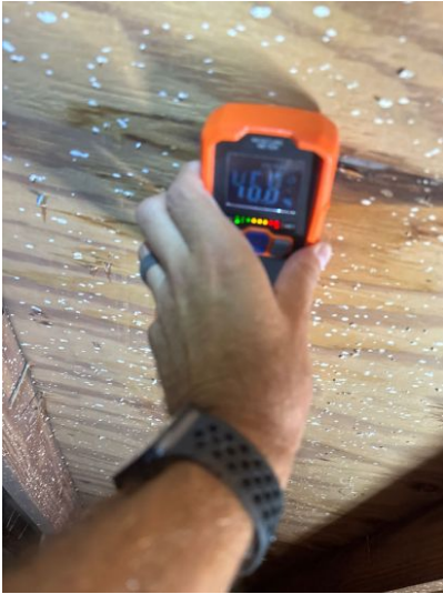
Unsatisfactory (attic water stain tested WET)
