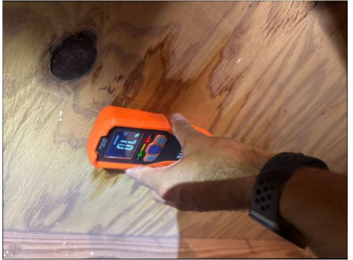
Unsatisfactory (attic water stain tested WET)
