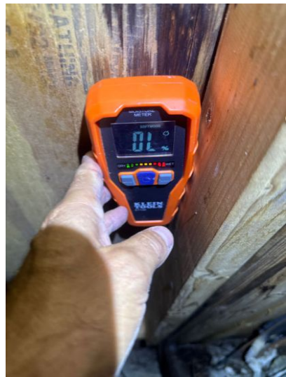
Unsatisfactory (attic water stain tested WET)
