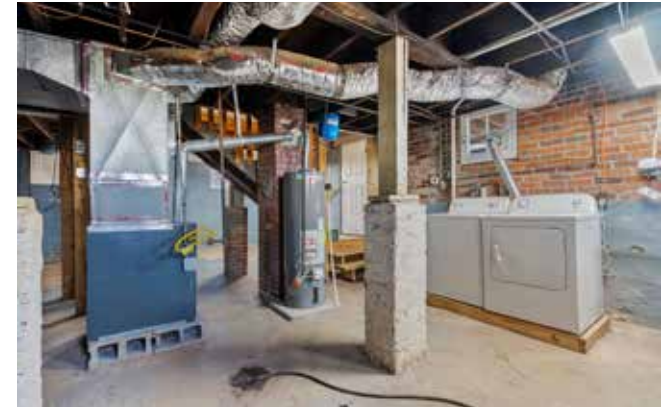
Basement Also Holds the Washer and Dryer
