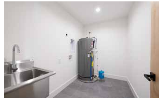
Upstairs Laundry Room • Heat Pump/Hot Water Heater
