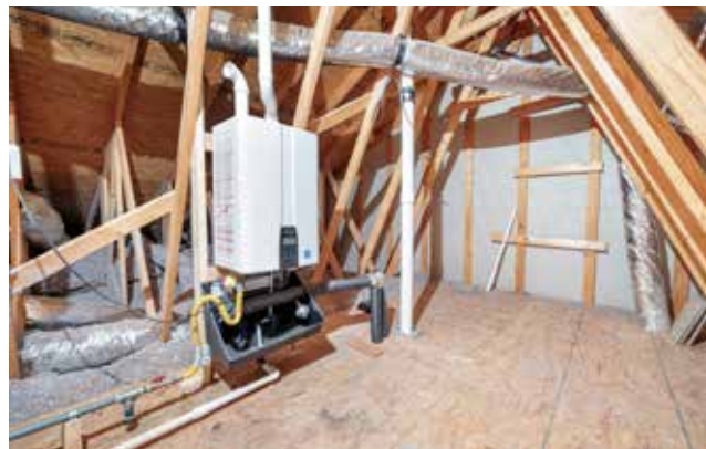
Amazing Attic Space and On-Demand Water Heater
