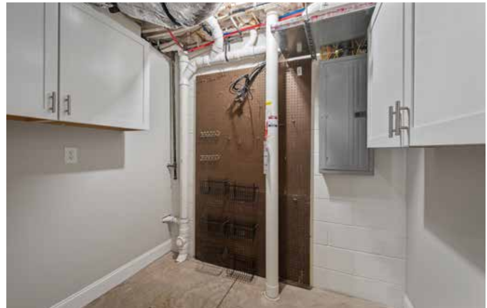
Tidy Mechanical Room
