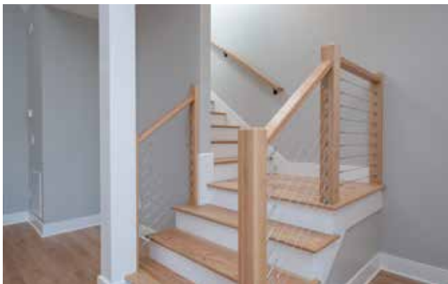
Cable Railing in Stairwell
