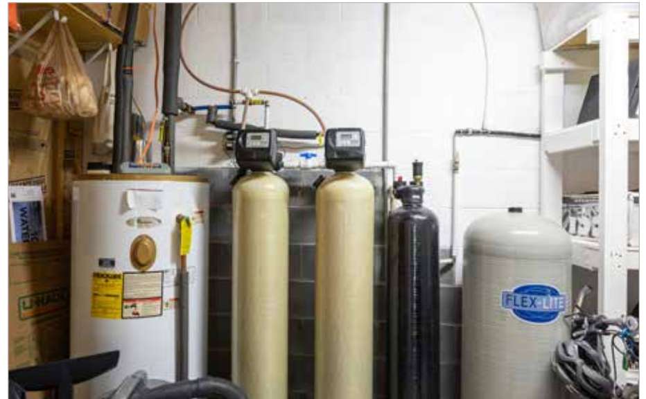
Wonderful Well Filtration System
