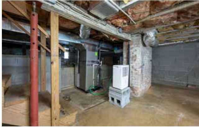
Downstairs, the Basement Has a Newer Gas Furnace ...
