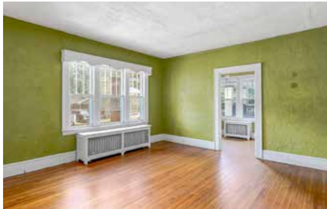
Steam Radiator Heat in Multiple Rooms
