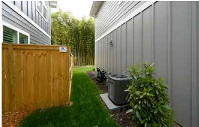
Two-Year-Old, Energy-Efficient HVAC System
