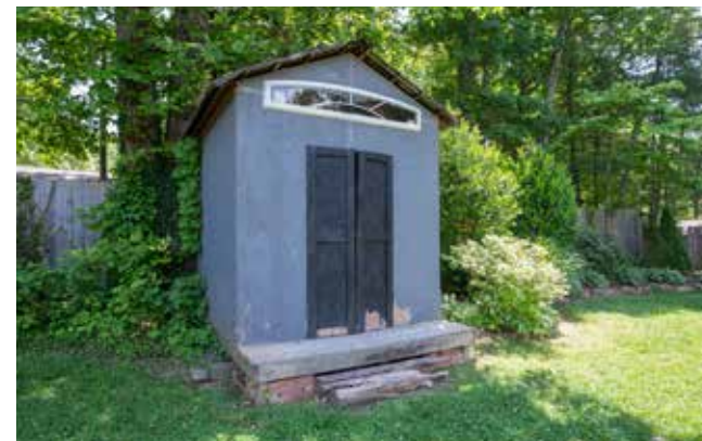
Rustic Shed (Needs Some Repair)
