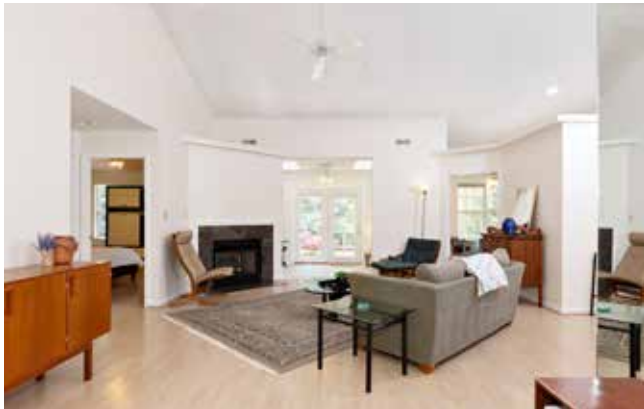
Natural Gas Fireplace in Living Room
