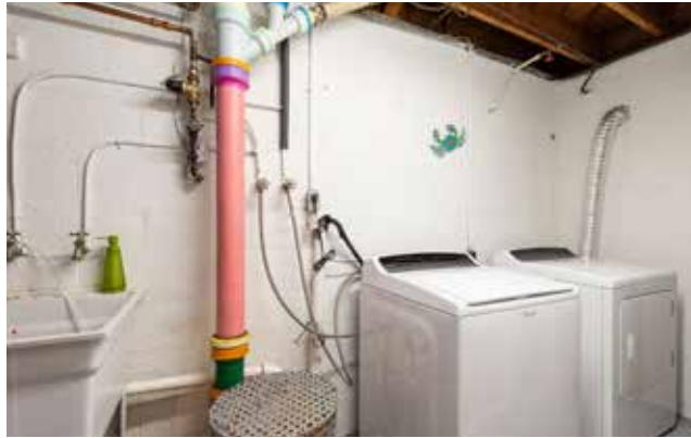
Washer and Dryer Located in Basement
