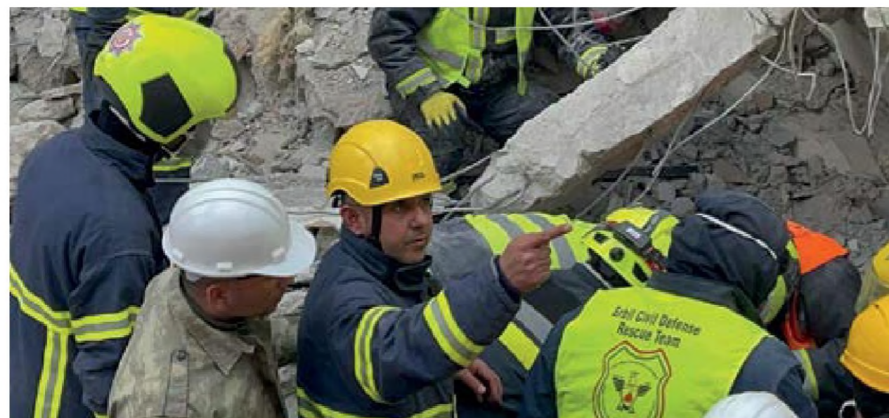
Kurdistan Region crew removing building rubble in the aftermath of the earthquake in Turkey.
