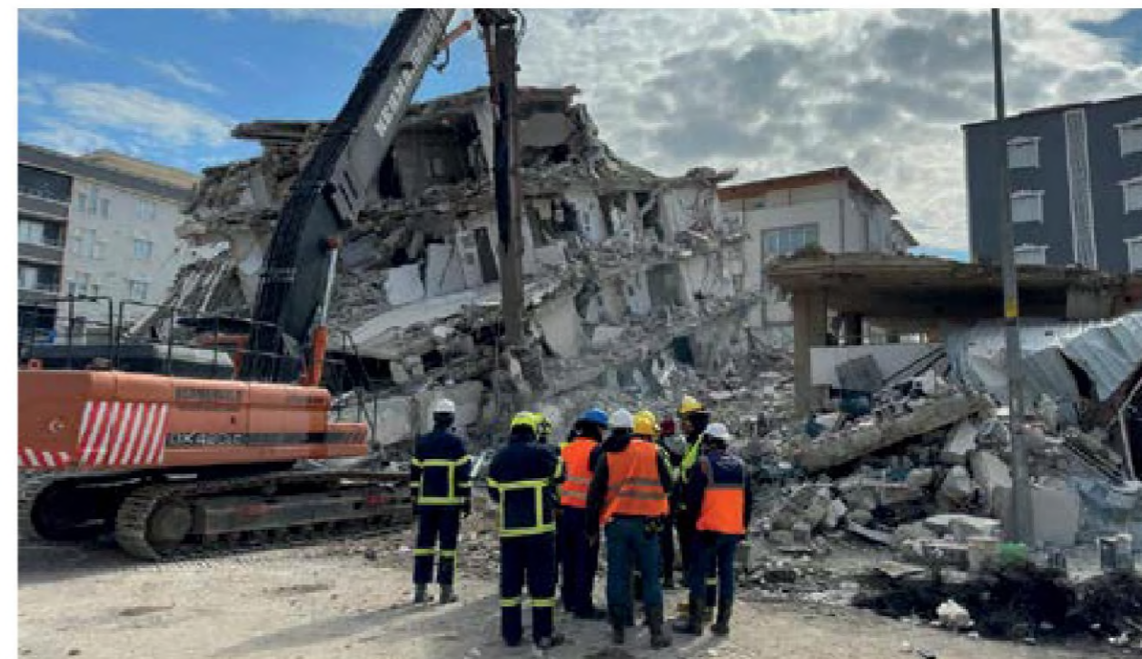
Kurdistan Region crew removing building rubbles in the aftermath of earthquakes in Turkey.
