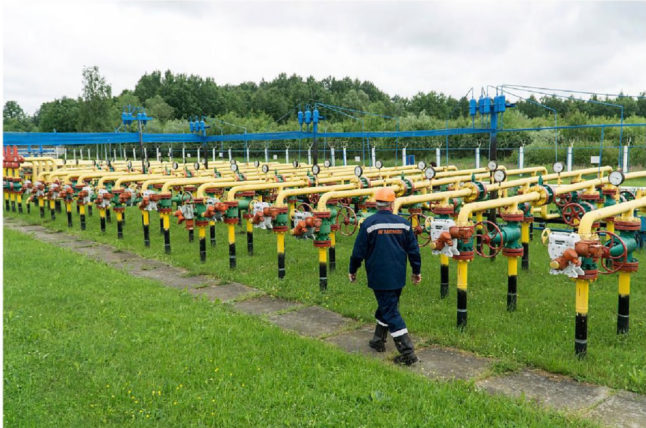
An employee from UkrTransGaz, part of Ukraine's state-oil giant Naftogaz, walks past gas pipes at the Dashava underground gas storage facility in Striy, Lviv Oblast on May 28, 2015. (Photo by Vincent Mundy/Bloomberg via Getty Images)
