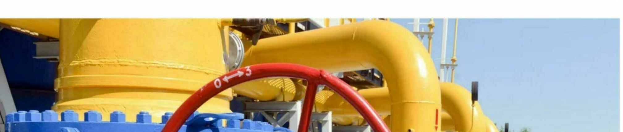
▲ Compressor station of Ukraine's Naftogaz national oil and gas company near the northeastern Ukrainian city of Kharkiv | Sergey Bobok/AFP via Getty Images
