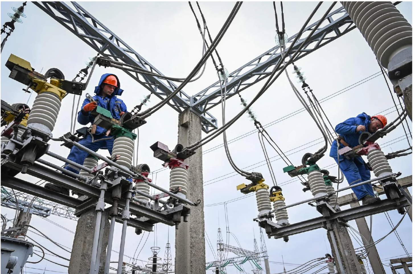
Moldovan electricians work on maintenance of energy infrastructure amid the Russian energy squeeze | Daniel Mihailescu/AFP via Privacy
